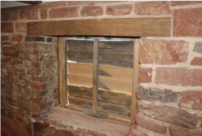
The simple but effective opening mechanism inside one of the louvers in the east wall. The handle turns the central pivot which opens each top hung slat together
