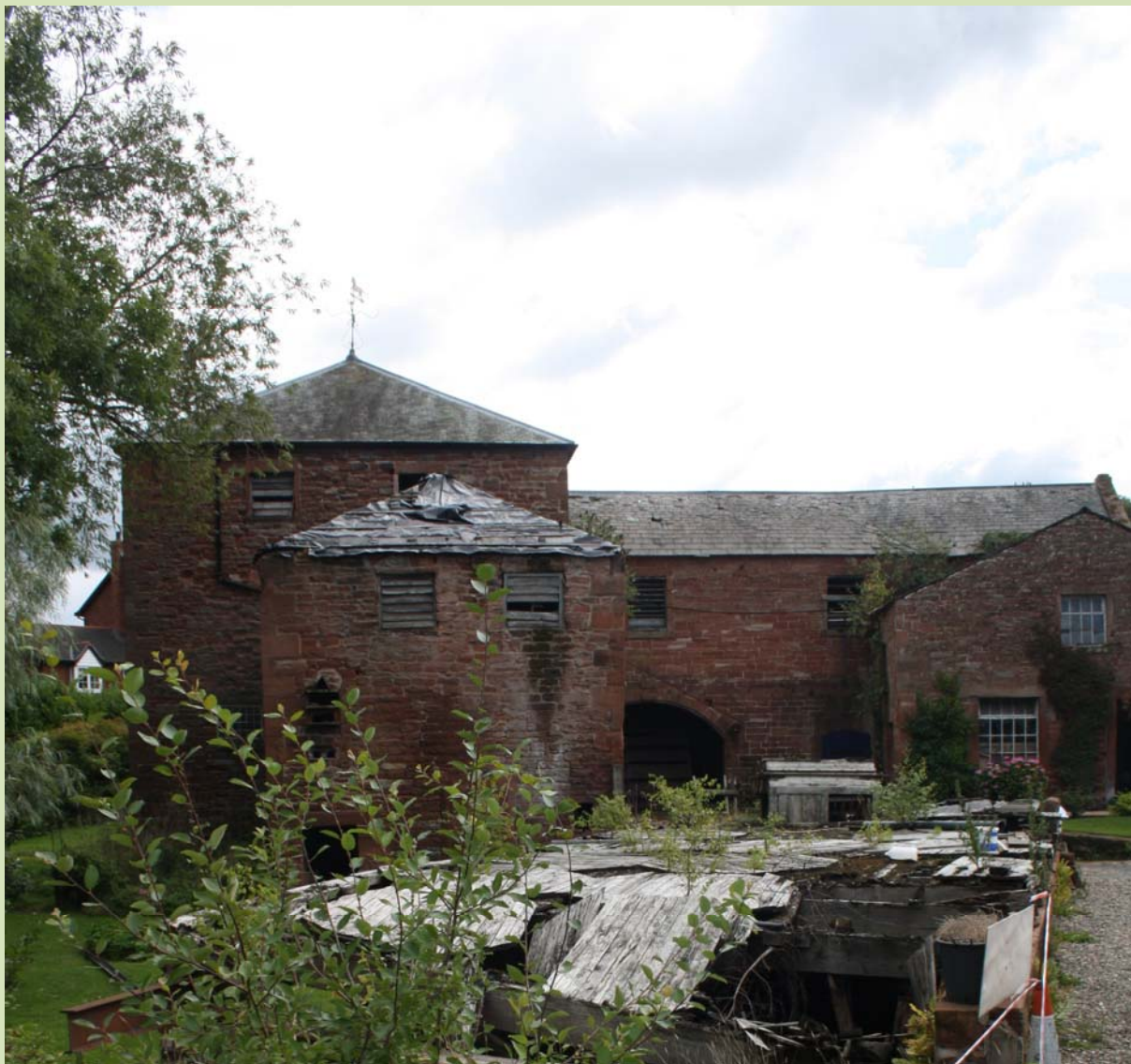
Warwick Bridge Corn Mill, Spring 2016 – the drying kiln roof protected only by plastic sheeting.
