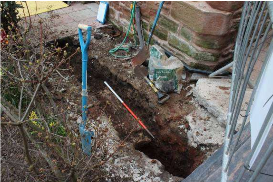
Wall foundation extending westwards from the south wall of the wash house
