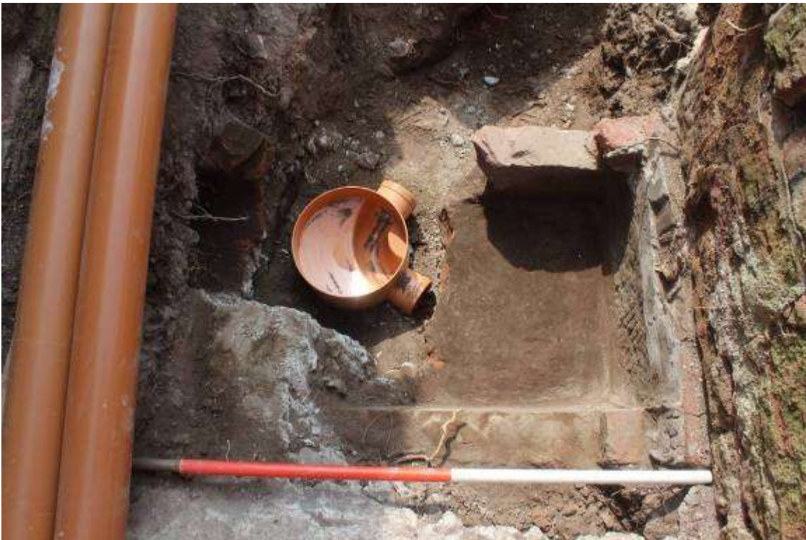
Removing the concrete ramp cut through the stone trough below the parapet wall of the eastern loading dock (right)
