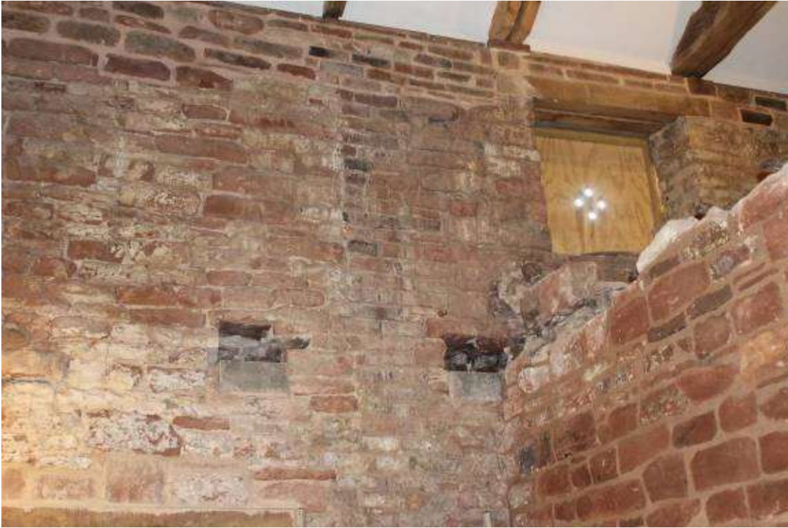
Slots in the south wall of the kiln for new padstones to support the new floor
