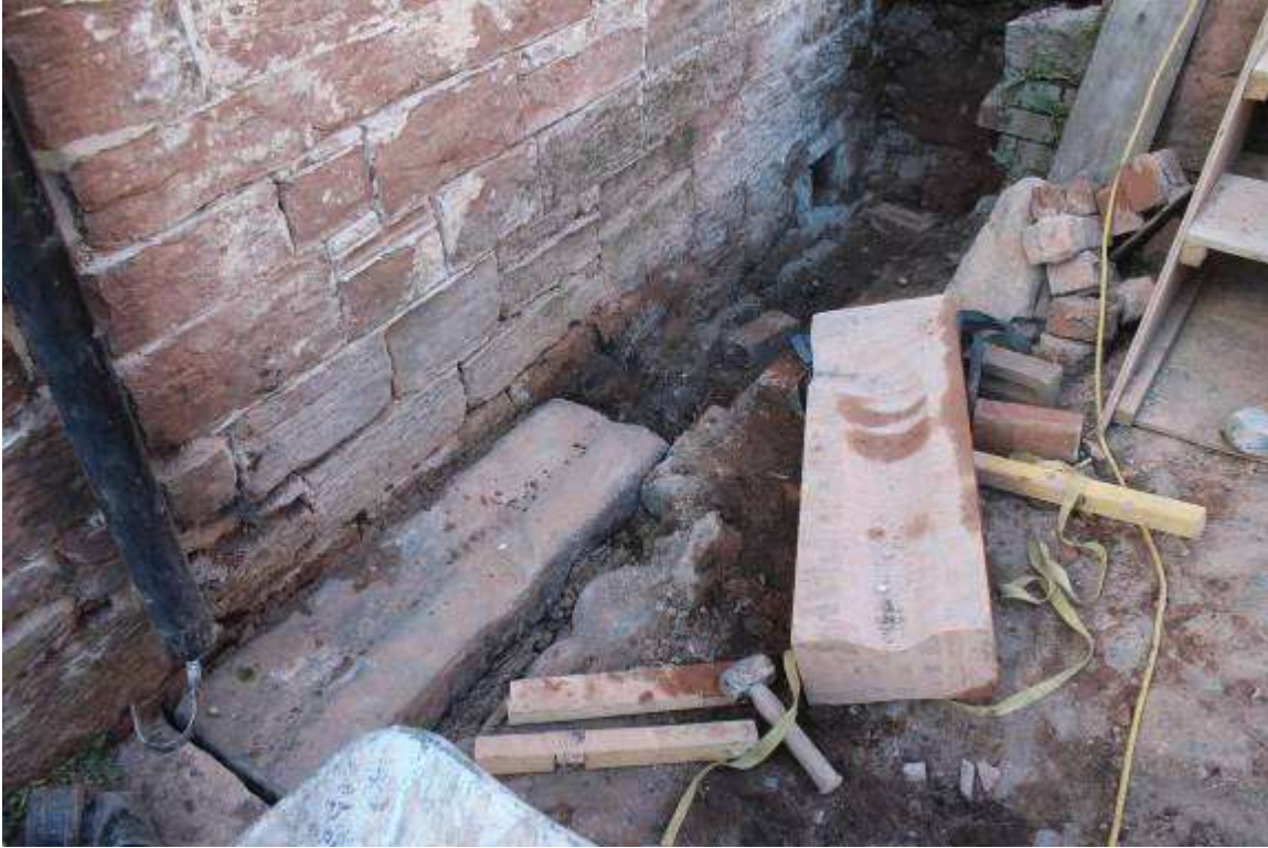
Resetting the drainage channel stones alongside the east side of the barn. A newly carved stone will turn the water into the old drain below the barn wall and into the wheel pit
