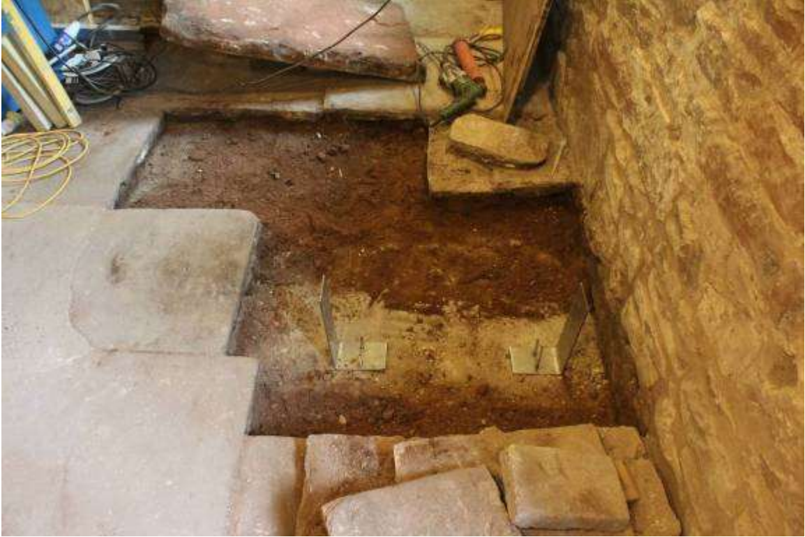
Repair underway to the Hurst Floor paving and new fixings for the staircase
