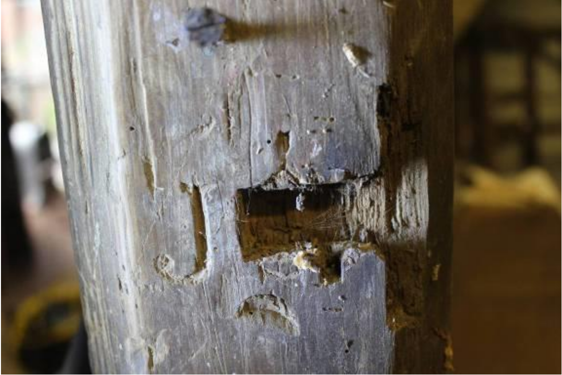
An earlier J, the rest of the initials perhaps removed by a later mortice, below on the same timber
