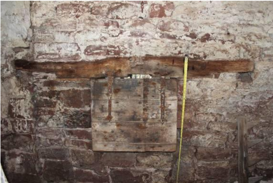
The shaped timber, with evidence of previous jointing, has been re-used to form the inner lintel of the hatch opening in the north wall of the chaff store
