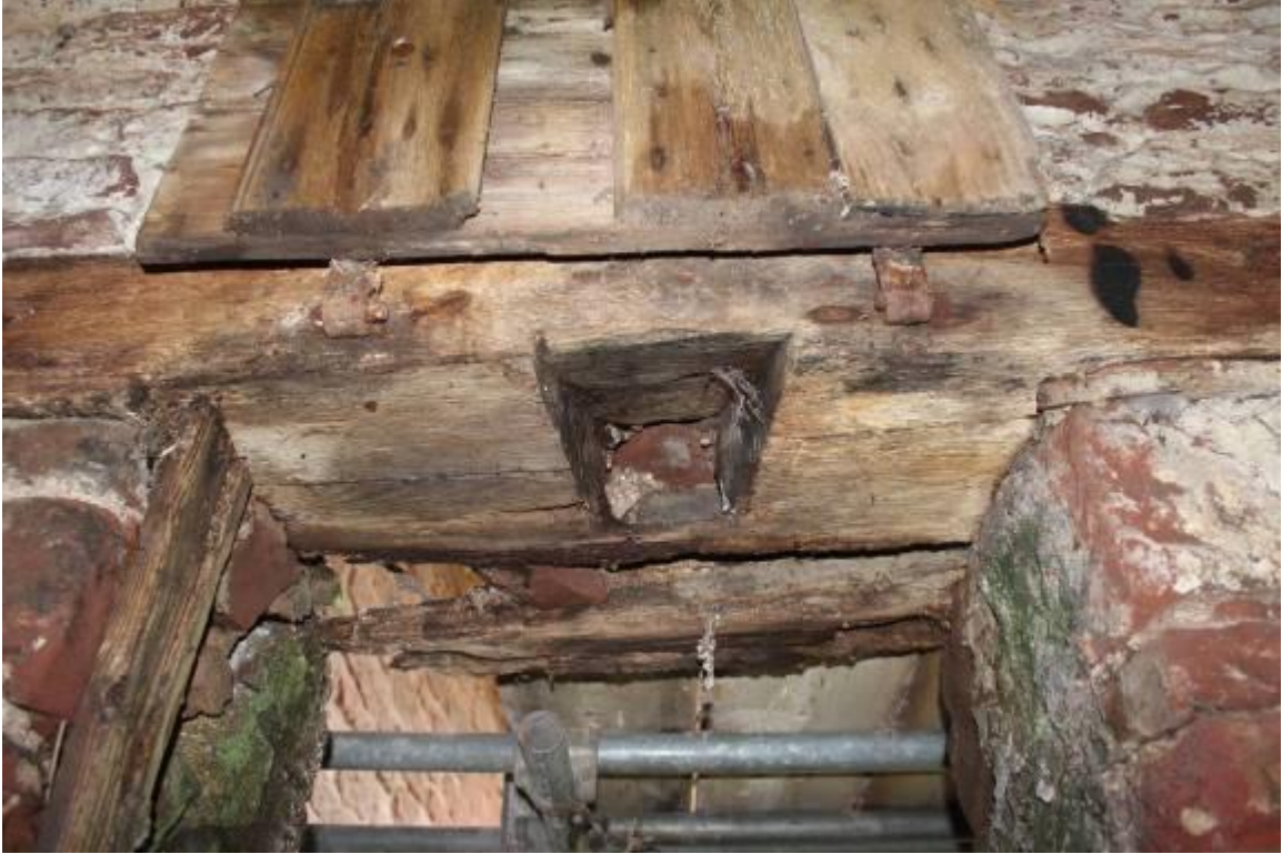
Angled mortice in the centre of the re-used timber. The outer timber lintel is almost rotted away
