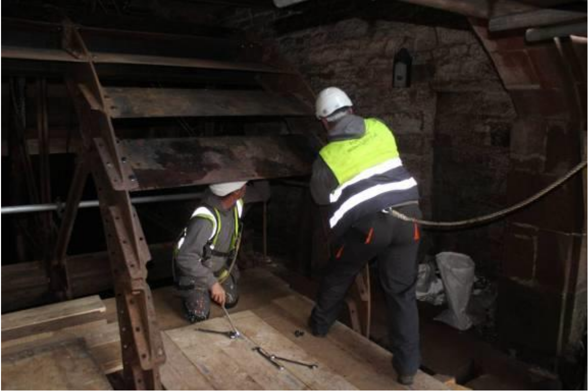
The millwrights installing new buckets on the south side of the wheel
