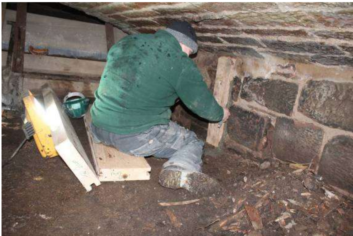
Pointing in a new timber for the box lining within the Head Race culvert
