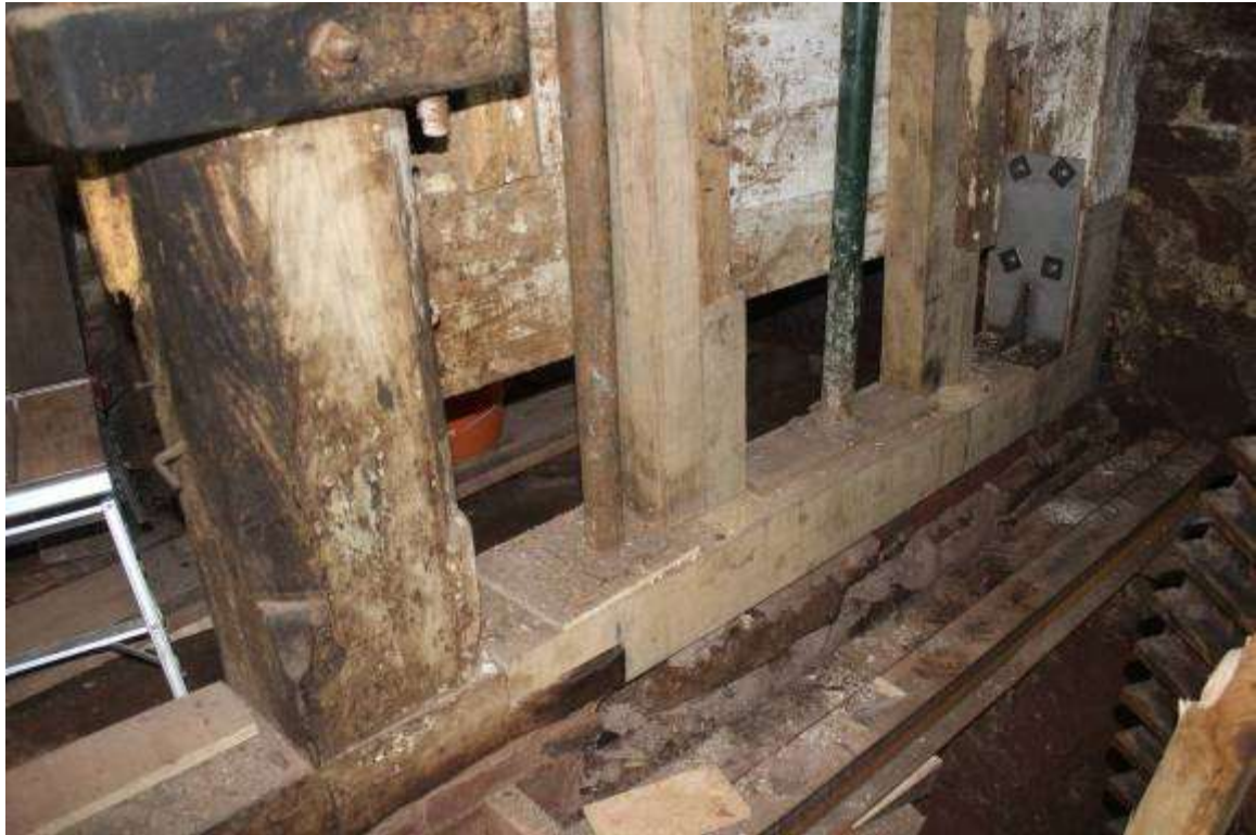
Repairs to the sill beam on the upstream side of the Hurst
