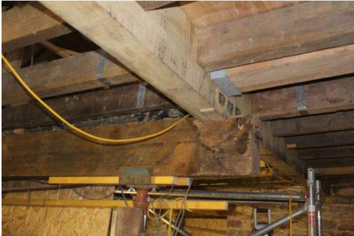
New Garner Floor Oak beam, installed in two lengths and plated together above the Bowstring Truss added by the Victorians to accommodate the fifth pair of millstones
