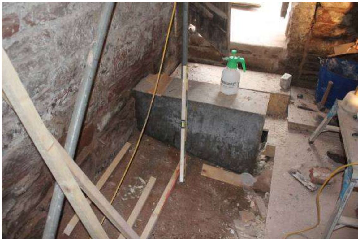
New support block for a staircase beside the drying kiln. The slope of the bedrock here is evident
