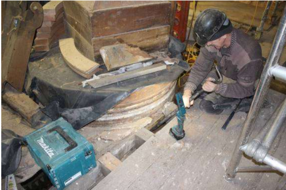
Digging out softened wood from the Stone Floor beam ahead of resin repairs
