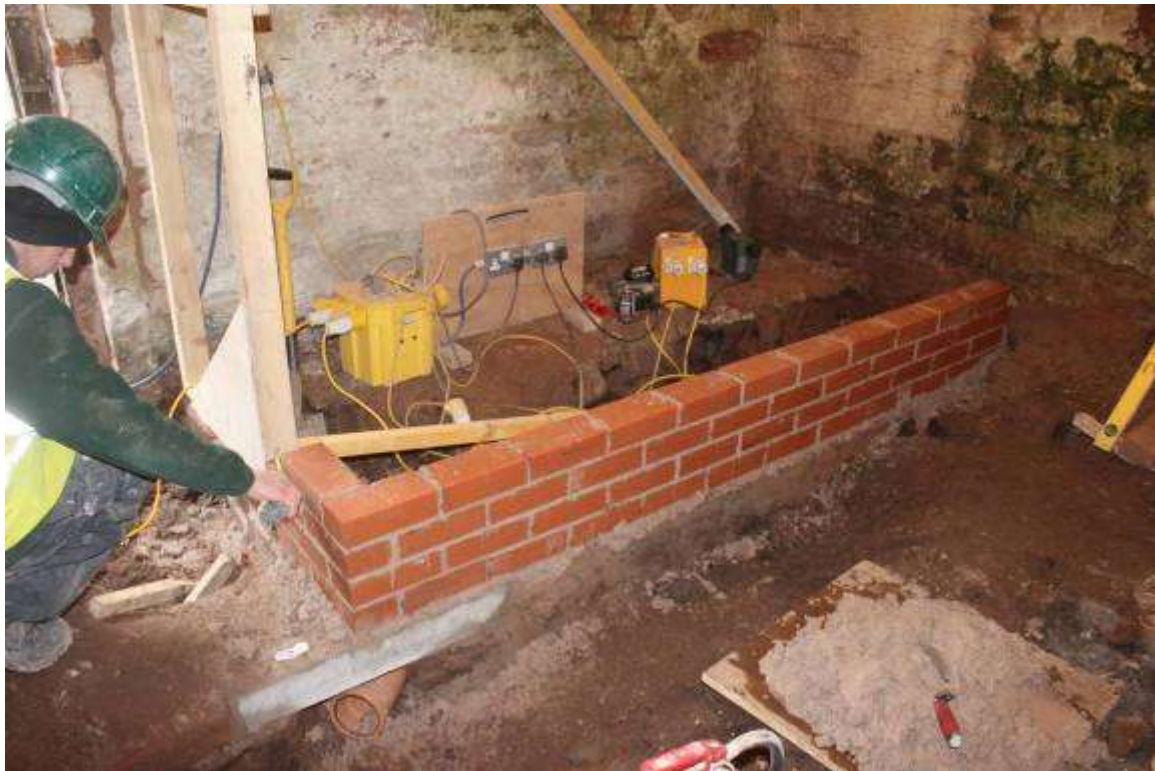
Partitions being installed over the earlier foundation in the ground floor Store
