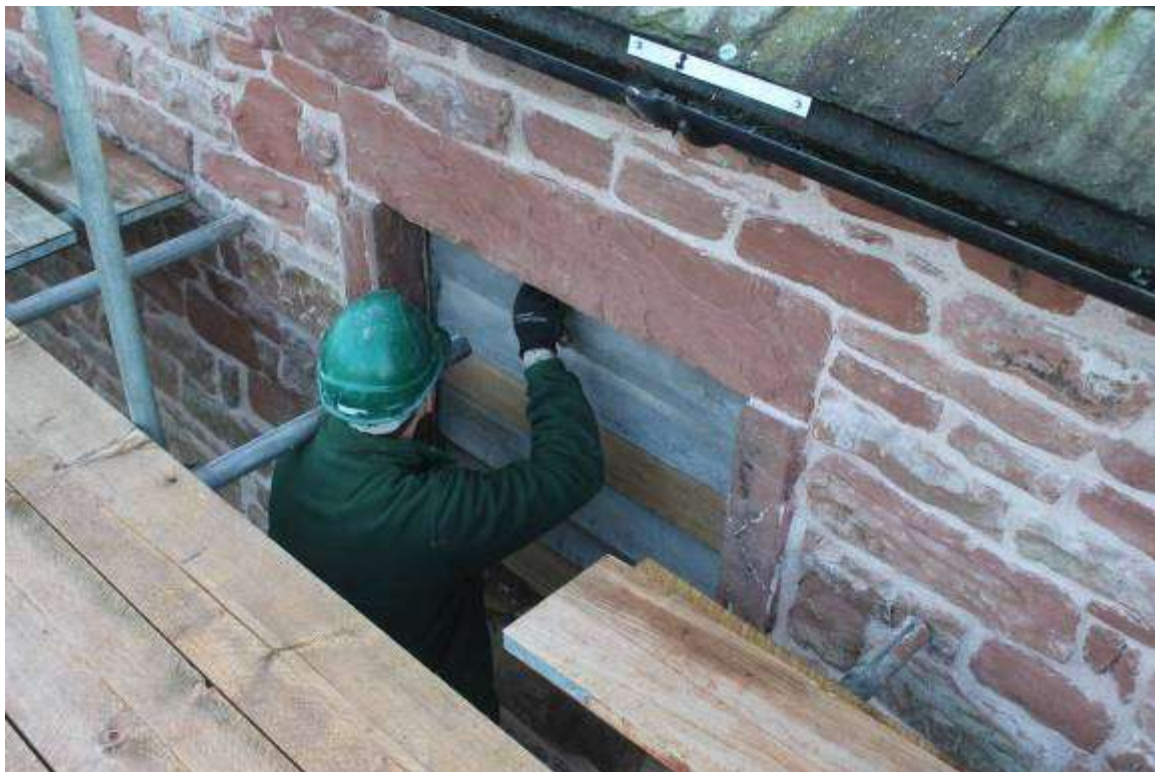
Pointing around a repaired louvre on the north side of the Garner Floor
