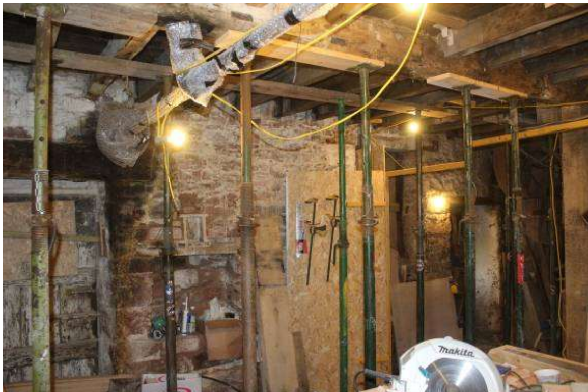
A double row of temporary props spanning the Hurst Floor are supporting the weakened Stone Floor beam
