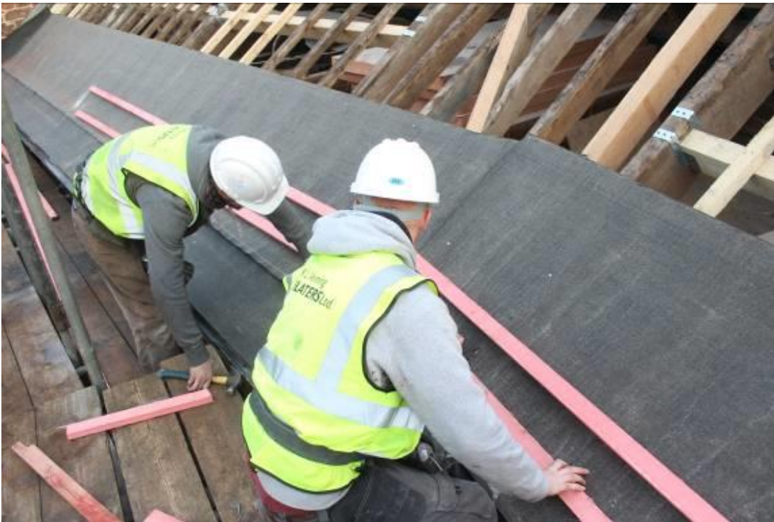
Work commencing on felting and fixing battens for the new slate roof for the barn
