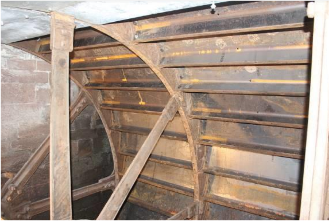
New buckets in place and sole plates, forming the inside of the buckets, partially completed (top left)
