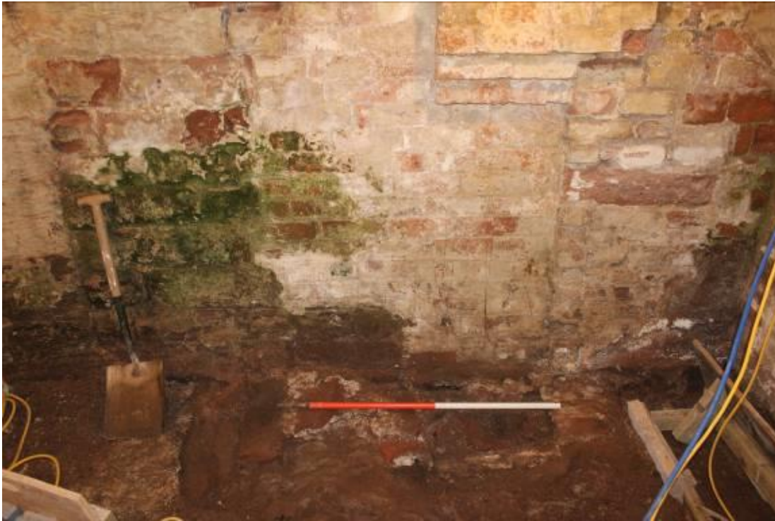
The base of a fireplace projecting below the brick blocking in the east wall of the store
