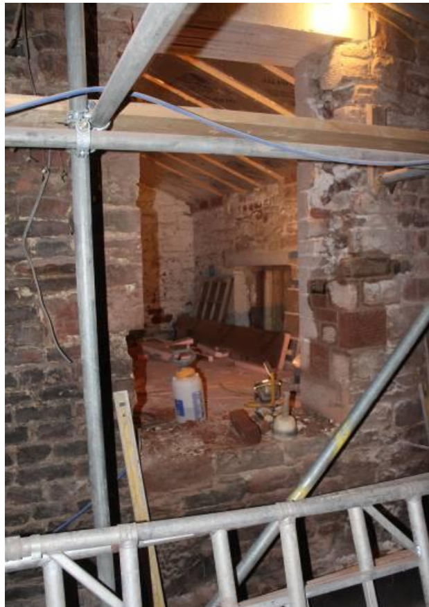
The blocking brickwork of the flue cut into the barn wall can be seen to the left of the new doorway
