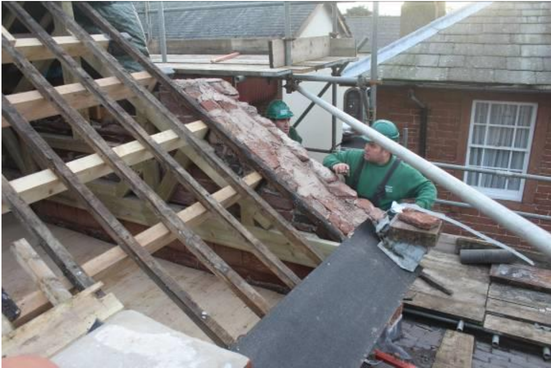
Sean, Site Manager, guiding consolidation work in progress on the south gable of the barn
